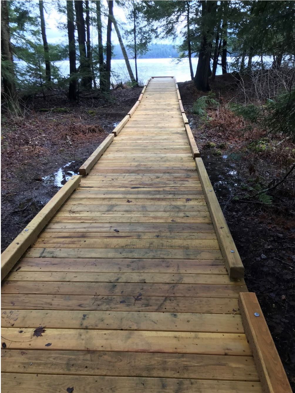
Figure 3. Sunset Lake (Benson) – This boardwalk is part of a newly constructed ADA accessible access area that was constructed on the north side of Sunset Lake. The project included significant upgrades to a camp road that leads to a new parking area which will serve both the fishing access area and Pond Woods Wildlife Management Area. From the parking area, there is a short gravel trail which leads to the boardwalk and lake shore where anglers and paddlers can access the lake.
