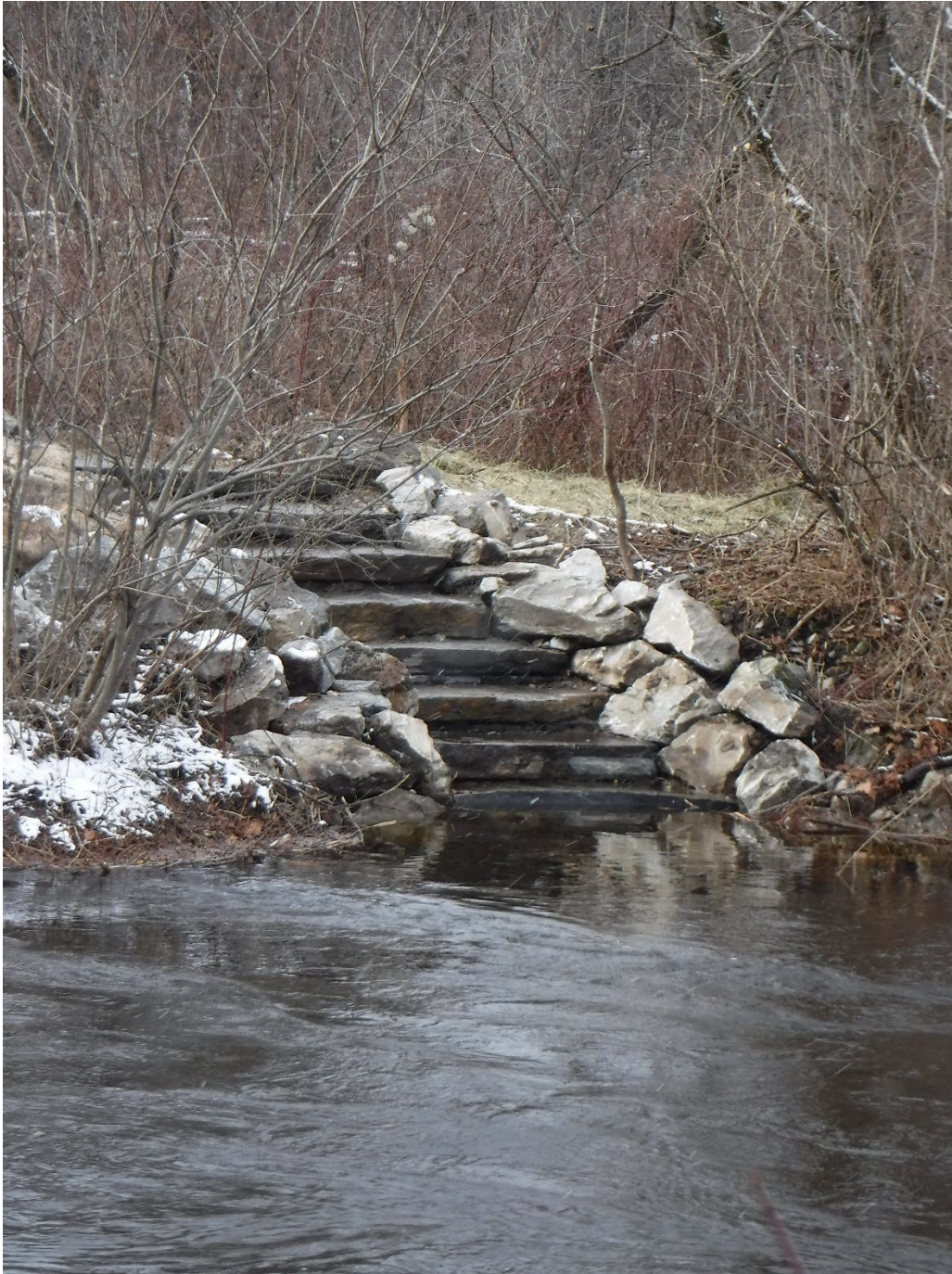
Figure 1. Otter Creek WMA (Mt. Tabor) – New stairs were installed on the WMA just east of Rt 7 to enhance fishing and paddling access to the creek. This site is extremely popular for both paddling and bank fishing. It is also a trophy trout stocking site.
