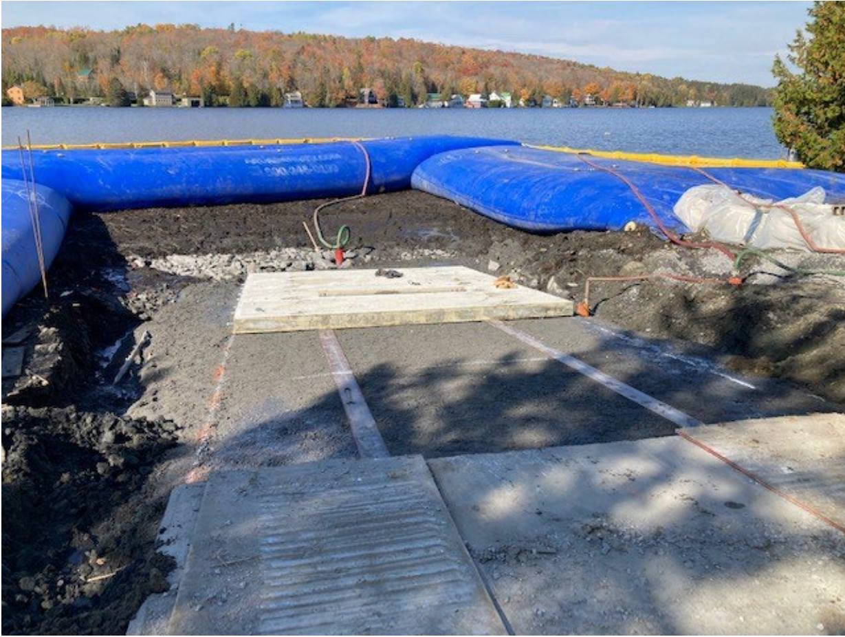
Figure 2. Joes Pond (Danville) – The existing ramp was shallow and had an 18-inch drop-off that was causing boaters to damage their trailers. A bladder dam was installed so the contractor could excavate the lake bottom to the appropriate grades and remove the lower portion of the old ramp before pouring the new concrete ramp. The rebuilt ramp is longer and deeper so it will provide boaters with a safer launching experience.
