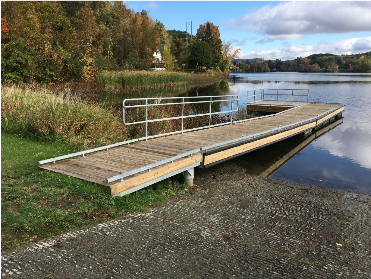
Figure 1. New dock and fishing platform at the South Bay Fishing Access Area in Newport, VT
