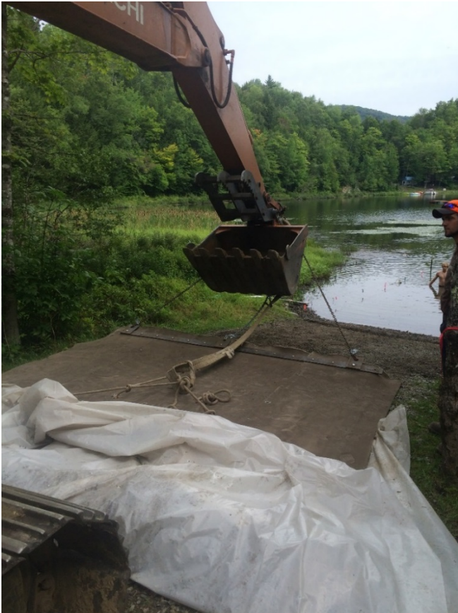
Figure 4. Concrete cloth being dragged into place on the gravel bottom of the Dog Pond Access Area, Woodbury, VT, August 2016.
