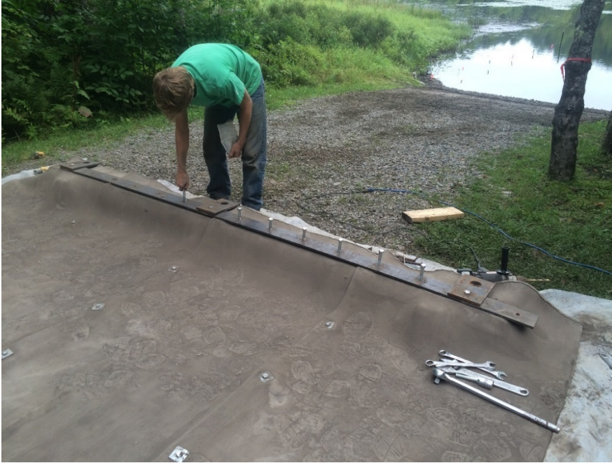
Figure 3. Bolting the 4 ft. strips of concrete cloth together prior to setting it in place at the Dog Pond Access Area in Woodbury, VT.
