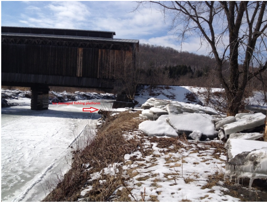
Figure 1. The 10x20 Fisher Bridge fishing platform on the Lamoille River in Wolcott was damaged following heavy February rains and subsequent flooding. Sheets of ice greater than 20 ft. across floated down the river, shearing off the platform's railing. The railing was replaced in June 2016.
